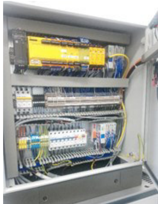
Fig. 9: Electrical cabinet of the safety PLC
