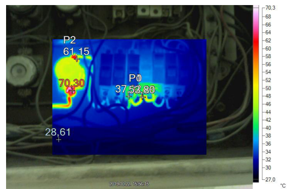
Fig. 4. Overheating lose connection
