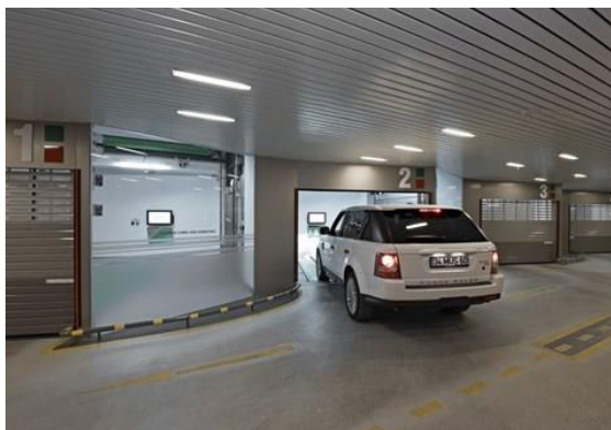
Figure 3. Entrance and exit of Robotic Parking Facilities [3]
