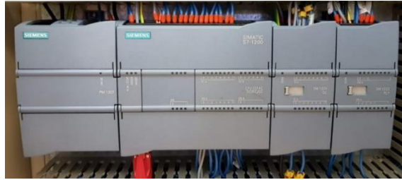
Figure 4. An S7 1200 PLC configuration: power supply, CPU 1214C DC/DC/DC, digital input and output extension modules
