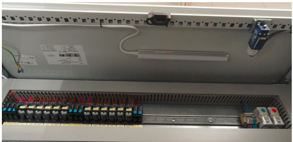
Figure 77 - Internal light and the first row from the top in F2 [33]
