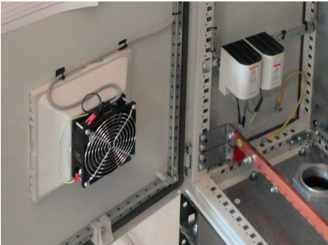
Figure 81 - Heating elements installed in the side of the control cabinet, and the cooling fan installed on the door of F2 [33]
