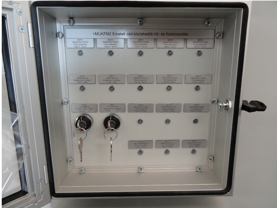
Figure 66 - Internal view of extra enclosure installed on the door of F1 [33]
