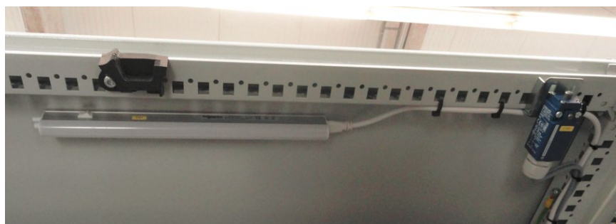
Figure 73 - The internal light and the switch that controls it [33]
