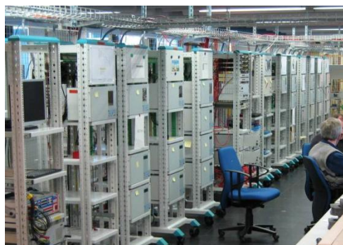
12. Figure Hitachi Energy Swiss test center
