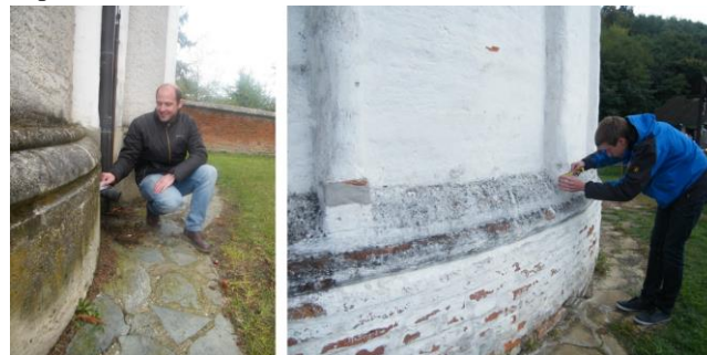
Figure 6. Good examples to right identify ground wall points at Ják (rough walling) and Kallósd (brick walling) church
