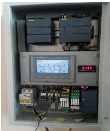
Figure 6. The appearance of the industrial controller unit
