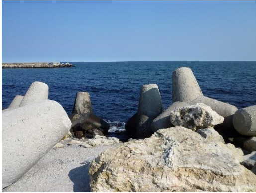
Figure 6. Broken tetrapod units
