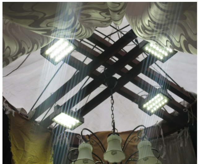
Figure 4. LED spotlights connected to low-voltage power supply system
