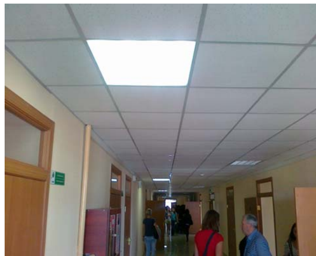
Figure 12. LED Lighting of the floor academic building
