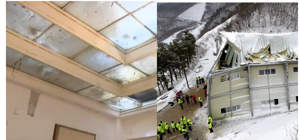
Fig. 3 Roof collapse due to the snow [ (a) Theatre in Czech Republic (b) University hall in South Korea]
