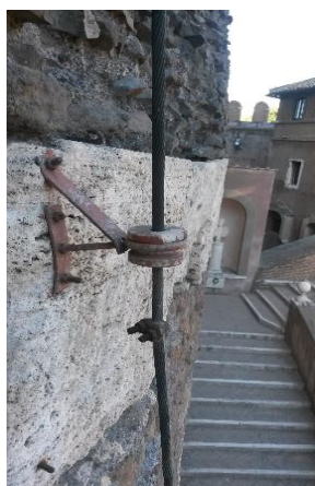
Figure 52: Lightning protection parts of cultural heritage building (Picture by author, 2017)
