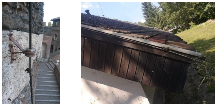
Figure 9: Rusted arrestors on different structures
