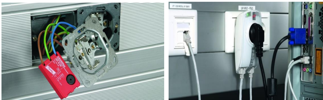
Figure 49: Installed overvoltage protection devices in use.
